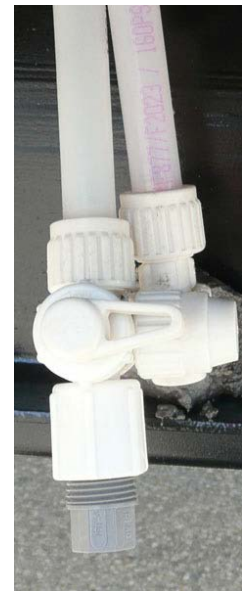
WATER TANK DRAIN VALVE
